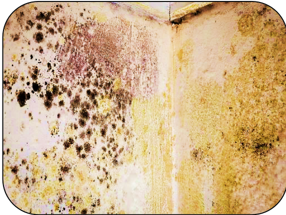
Fig. 6. Penetrating dampness connected to water intrusion into a wall element
