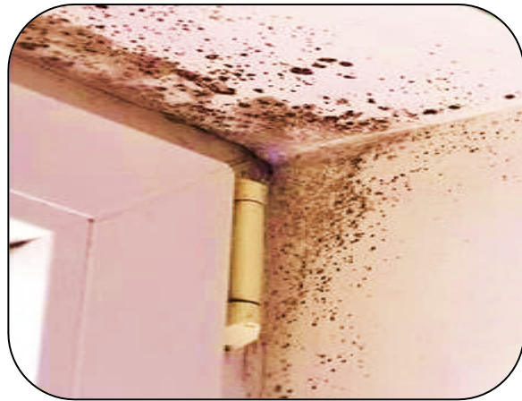
Fig. 5. Rainfall that hits the exterior walls and parapets caused falling dampness to occur
