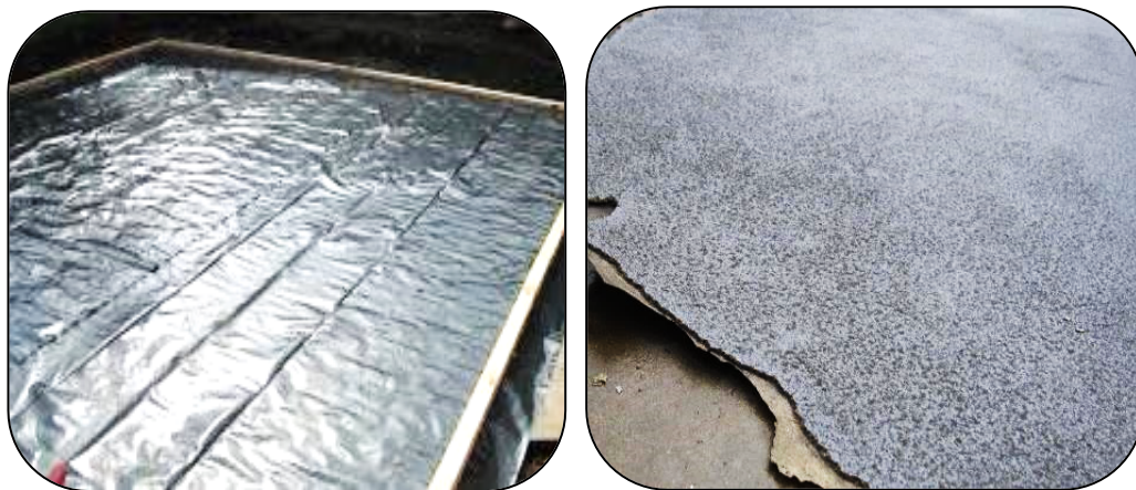
Fig. 13. Defective waterproofing membrane
