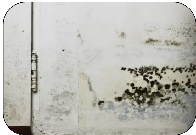
Fig. 7. Presence of black mold on internal wall surface
