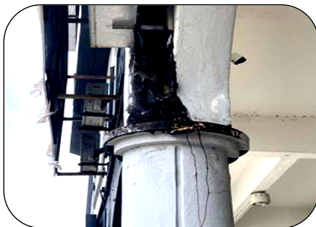
Fig. 8. The presence of fungus and moss in moist environment would gradually lead to erosion
