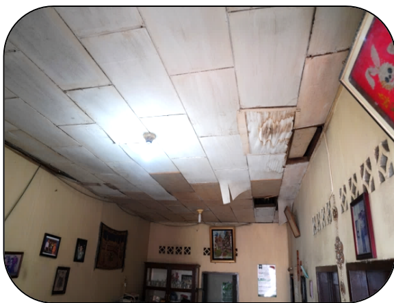
Fig. 10. Water seeping through the ceiling
