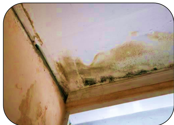
Fig. 11. Seepage resulting from breaches in the flooring
