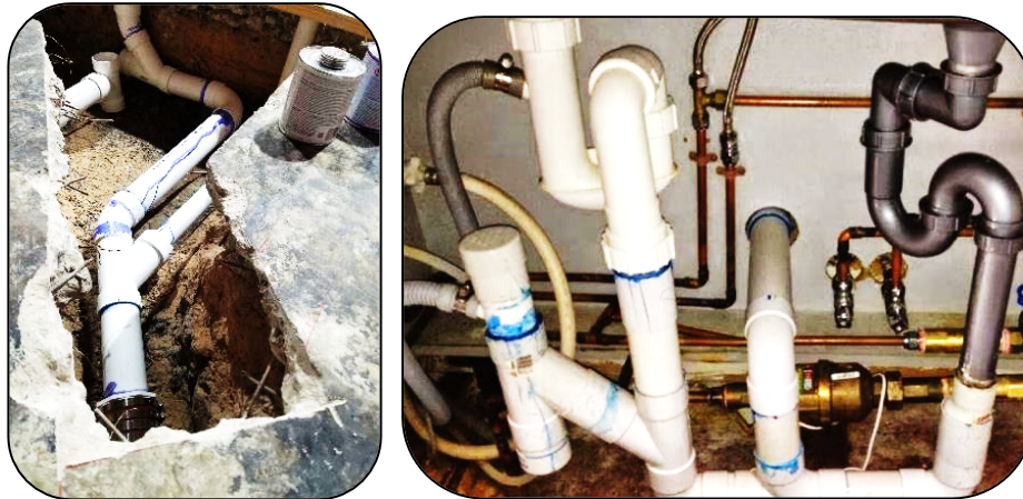
Fig. 14. Improper installation of plumbing
