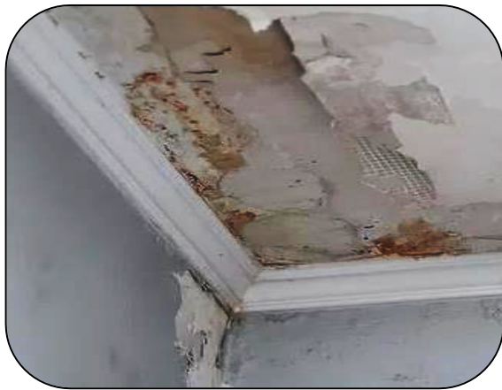
Fig. 4. Falling dampness occurred due to improper rainwater pipe connections
