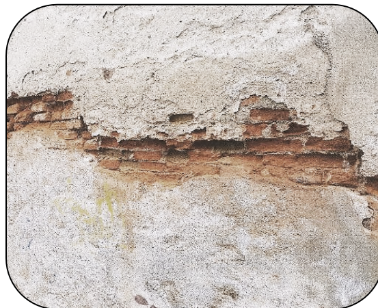
Fig. 3. Rising dampness occurred at external wall
