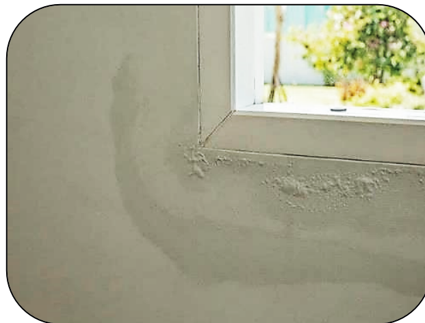
Fig. 17. The intrusion of rainwater through window and wall
