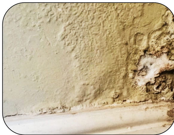
Fig. 1. Indications of rising dampness appear at the ground level
