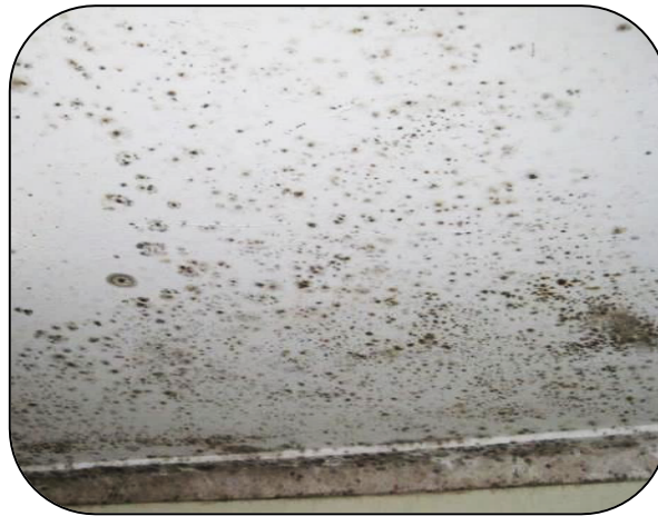
Fig. 18. Presence of dampness and mold growth due to inadequate ventilation
