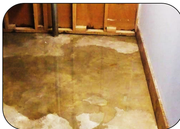
Fig. 12. Water seeping through the floor
