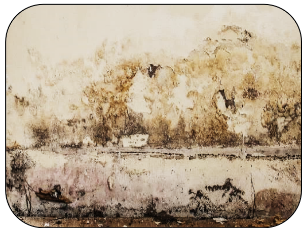
Fig. 2. A serious dampness problem occurred at the internal wall
