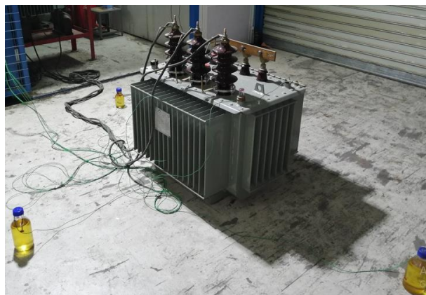
Fig. 4. The electrical transformer during the testing process
