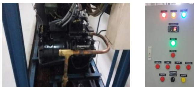
Fig. 11. Digital Compressor Rack with Distal compressor and digital controller
