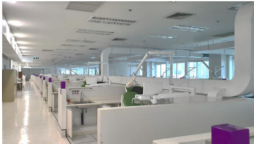
Fig. 1. Photo of air-conditioned clinical space of 50 multi-unit dental school in this study
