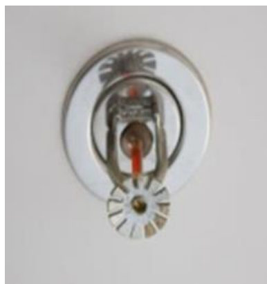
Fig. 1. The fire water sprinkler
