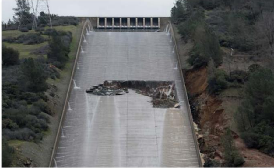
Fig. 2. Damage in Oroville dam spillway, causes by cavitation in California, USA [6]
