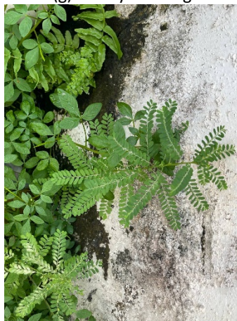
(j) Vegetation Encroachment
