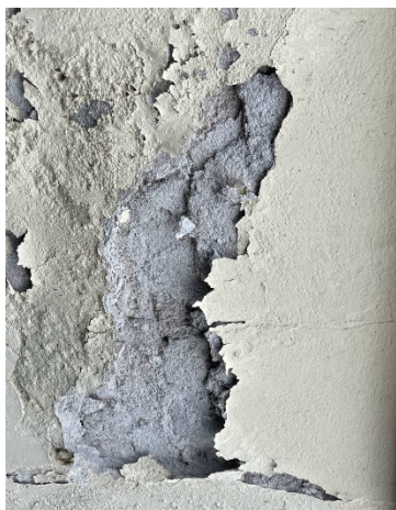
(a) Major cracks
