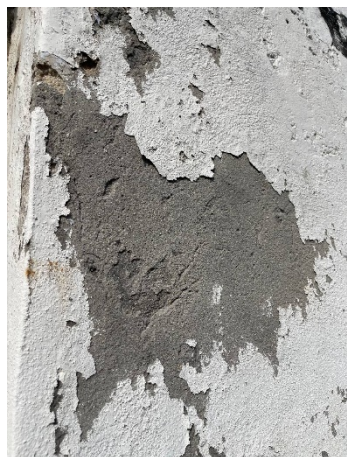
(b) Peeling Paint
