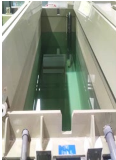
Fig. 2. Chemical cleaning tank
