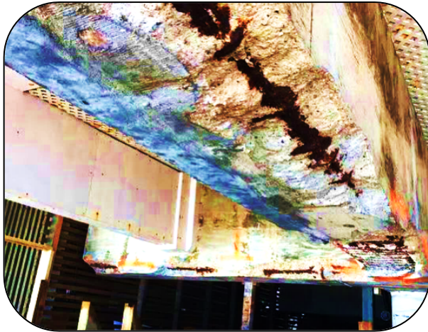
Fig. 9. Structural degradation impacting the stability and security
