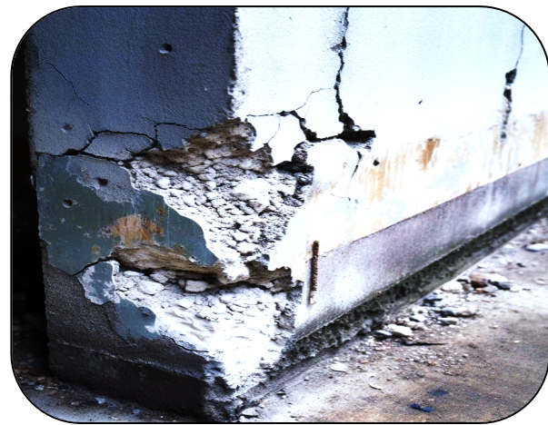
Fig. 10. Indication of concrete spalling observed on the wall
