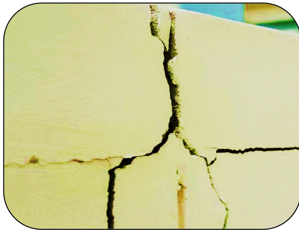
Fig. 7. Structural damage due to earthquake
