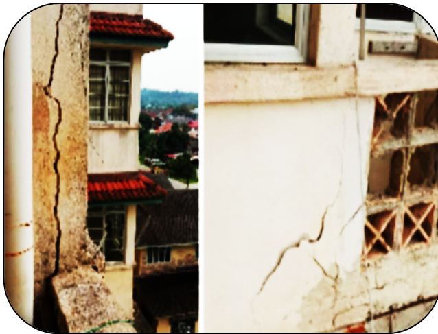
Fig. 4. Major cracks due to lack of project auditing
