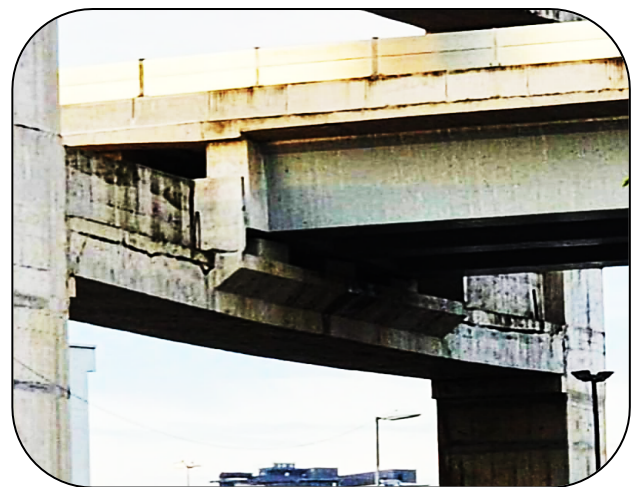
Fig. 5. Visible cracks highway structure
