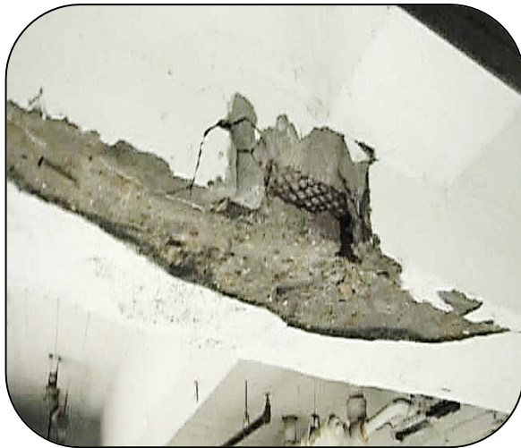
Fig. 2. Major structural cracks
