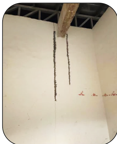
Fig. 8. Cracks appearance on wall surface
