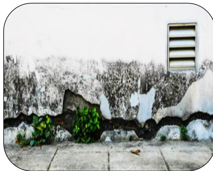
Fig. 10. Visible sign of sinking
