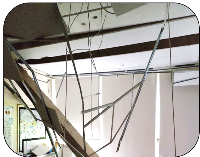
Fig. 3. Roof structure collapse
