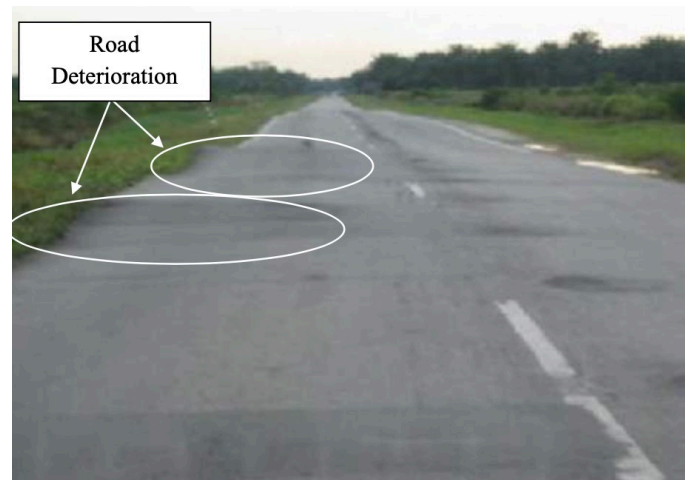
Fig. 1. Bulging along Pontian Road
