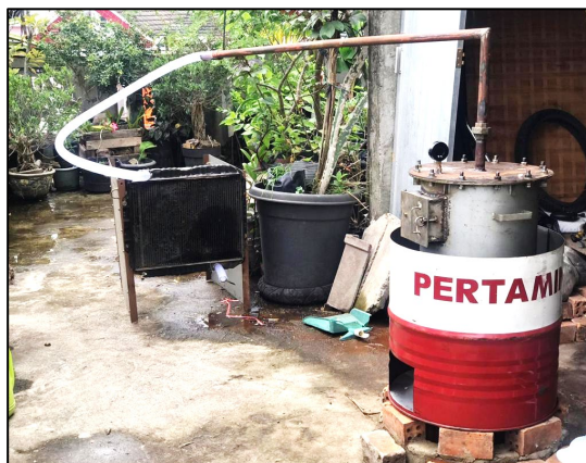
Fig. 2. Pyrolysis equipment sets [3]
