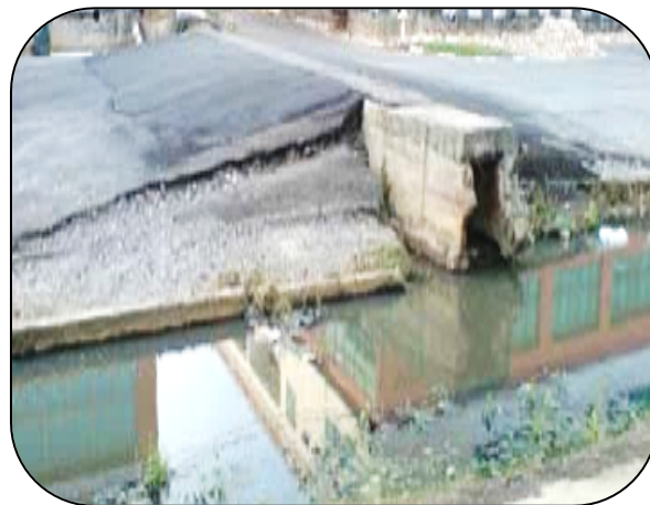
Fig. 18. Improper drainage and roadways may result in ground settlement
