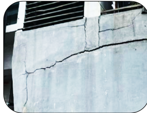
Fig. 5. Crack on shop lot structure
