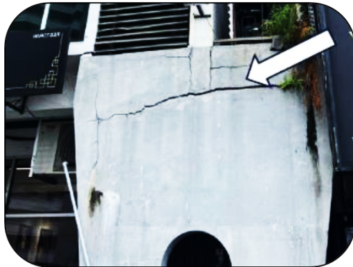
Fig. 4. Differential settlement at shop lot
