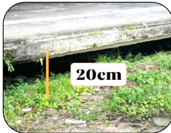
Fig. 12. Ground subsidence within the building
