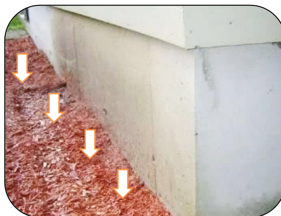
Fig. 17. Inadequate soil preparation may lead to settlement
