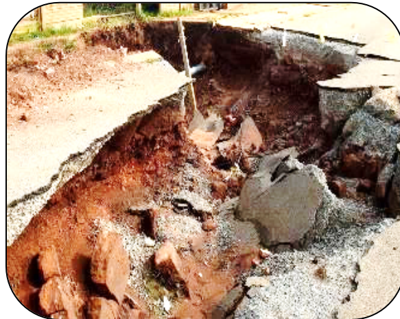
Fig. 20. Sinkholes may lead to settlement
