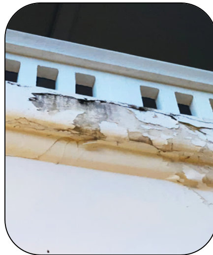
Fig. 2. Crack and dampness on the balcony
