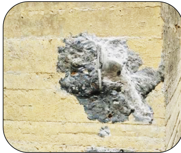
Fig. 5. Concrete surface deterioration
