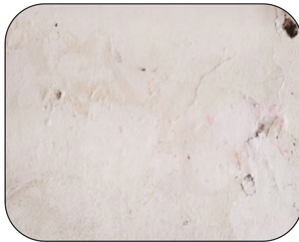
Fig. 7. Blistering on wall
