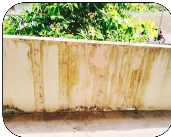
Fig. 3. Visible sign of dampness on external wall
