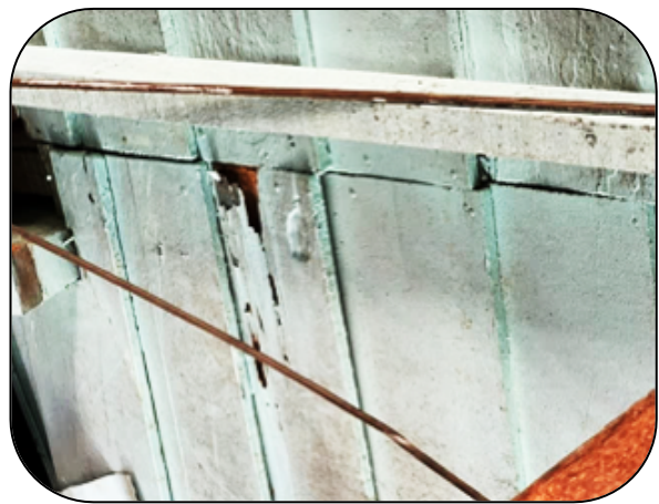
Fig. 3. Termite attack of timber wall
