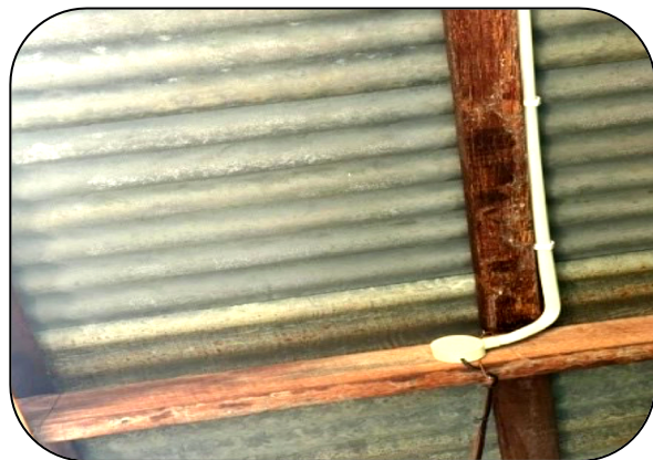
Fig. 7. Damage due to carpenter-ant attack
