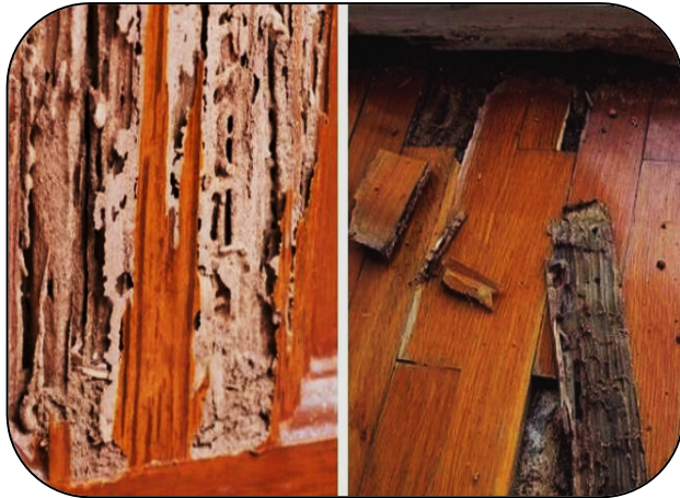
Fig. 2. Termite attack on wooden flooring
