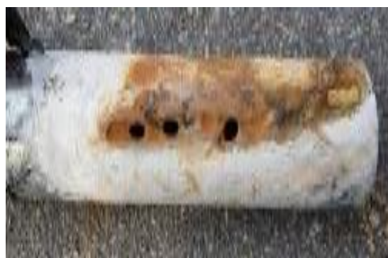
Fig. 1: The external corrosion of underground GI pipe
