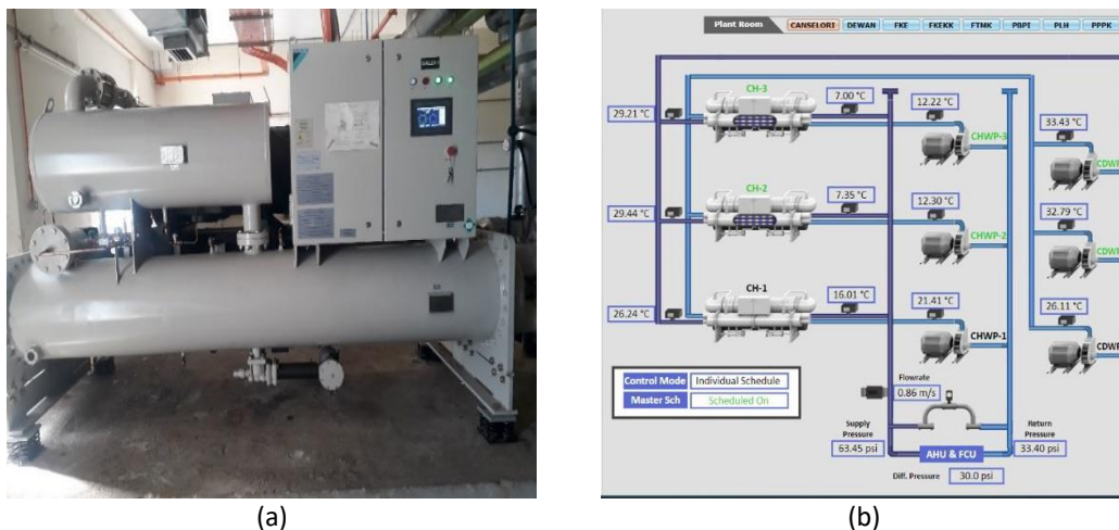
Fig. 4. Chiller System. (a) Picture of the retrofitted chiller at management building; (b) Chillers configuration that has been monitored through BMS system
