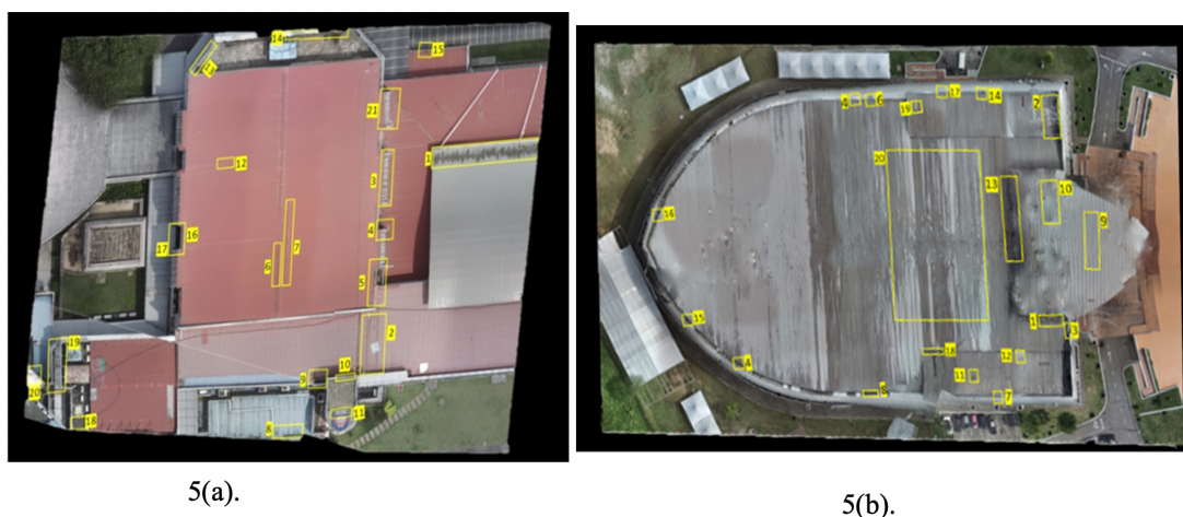
Fig. 5. (a) and (b). Full view of DSI and DTMI with the location of the defect
