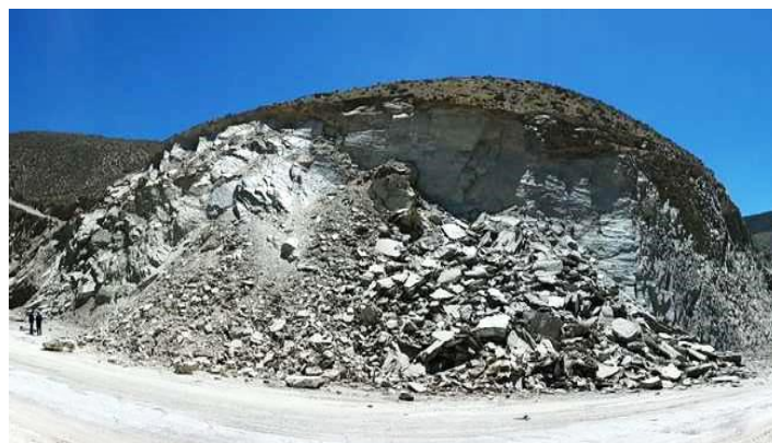
Fig. 3. Excavation of schist rock cut along the Taza-Hoceïma expressway on the National Road N° 02
