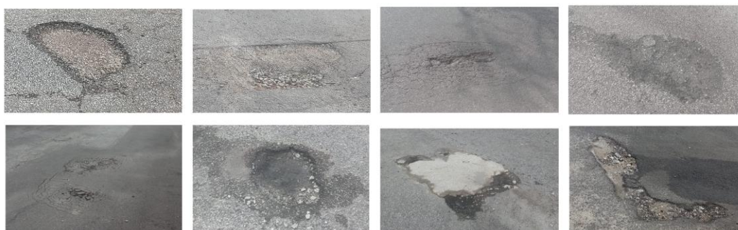
Fig. 4. Example of potholes measured during experiments
