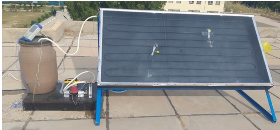
Fig. 1. Photograph of solar flat plate collector (SFPC)
