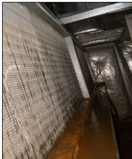
Fig. 1. Condensation in air handling unit
