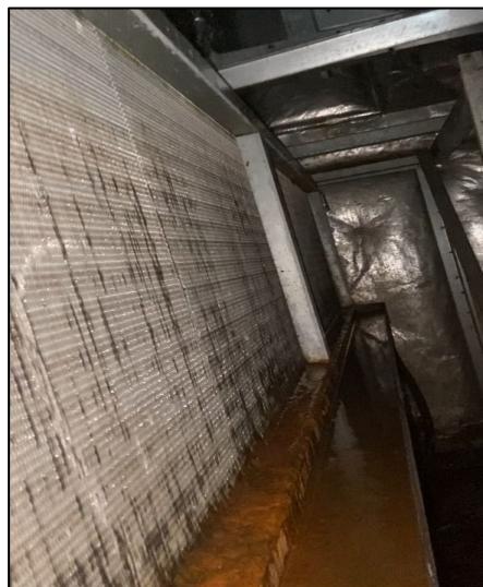
Fig. 1. Condensation in air handling unit
