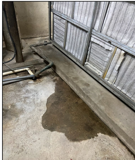
Fig. 2. Water leaking from air handling unit
