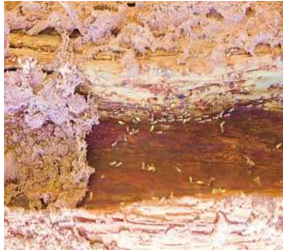
Fig. 8. Terminate attack on the timber flooring of a structure
