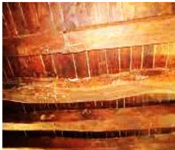
Fig. 7. Timber brittleness in the floor joist's section
