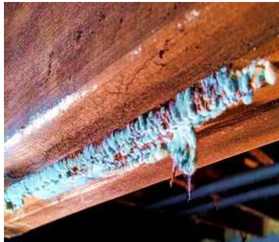
Fig. 6. Mould growth at timber structural beam
