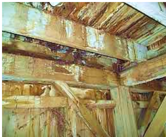
Fig. 2. Serious deterioration of structural timber
