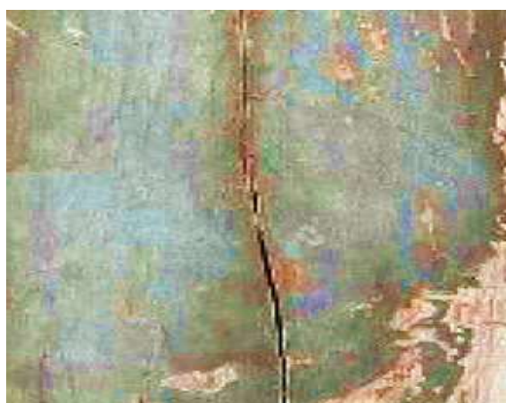
Fig. 3. Visible cracks on timber structure
