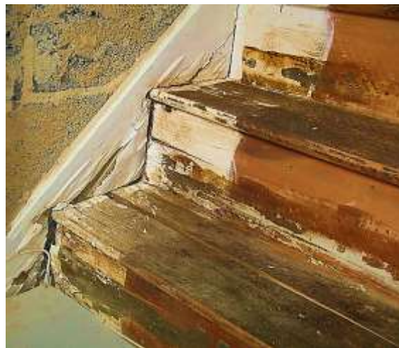
Fig. 1. Timber decay occurs at the staircase
