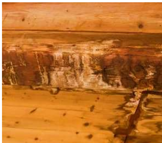
Fig. 5. Dampness problem on structural timber
