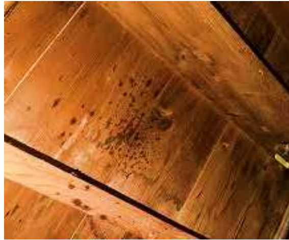
Fig. 4. Visible cracks on timber structure
