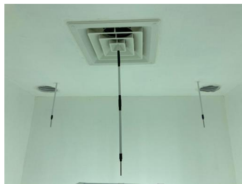
Fig. 3. The installation of the square diffuser and thermocouple type-K in the chamber
