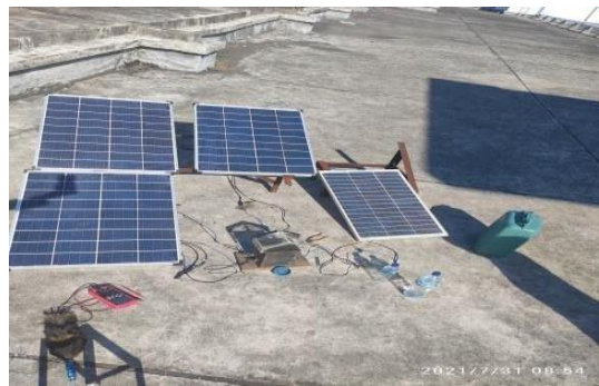
Fig. 4. Overall part of the distillator prototype installation
