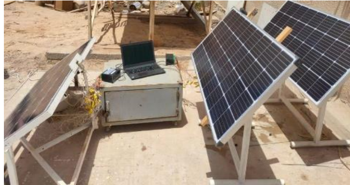
Fig. 2. Experimental structure of the PV modules
