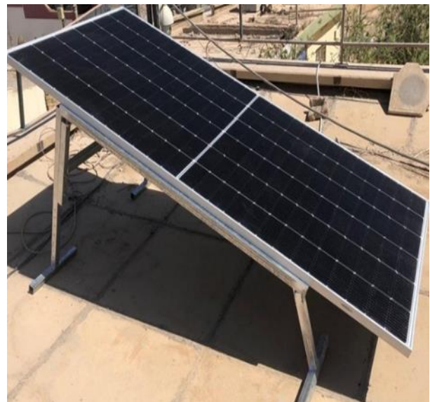
Fig. 7. Photovoltaic panel, nominal power 580W
