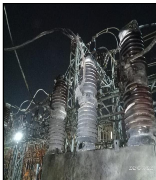
Fig. 3. Flashover from limb to mechanism
