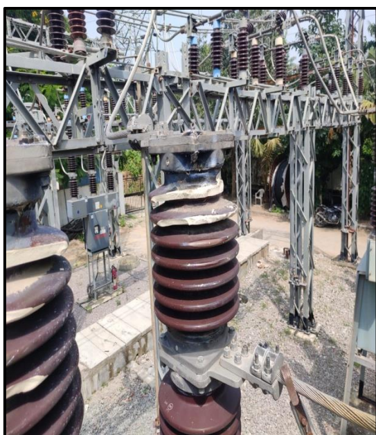
Fig. 2. Circuit Breaker limb flashover
