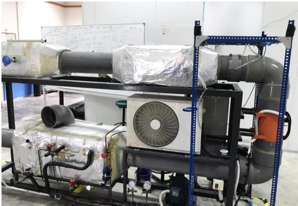
Fig. 1. HVAC experimental rig in Heat Transfer Laboratory
