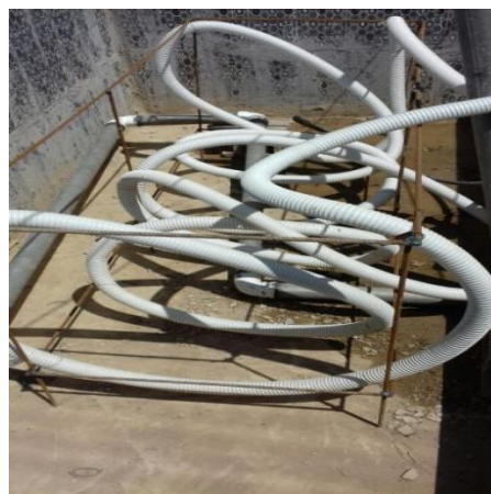
Fig. 1. Heat exchanger tubes (plastic)
