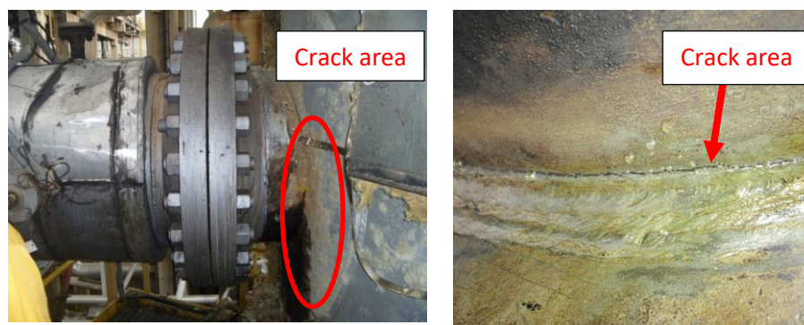
Fig. 1. Quench tower inlet nozzle N5 crack (in circle) at 180 deg location
