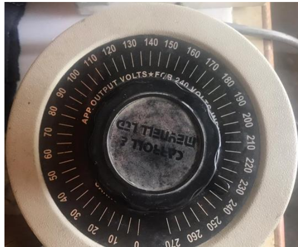
Fig. 22. Voltage supply transformer at 150V
