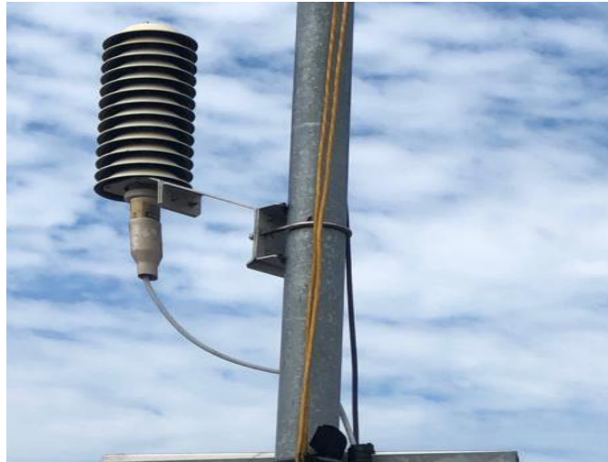
Fig. 4. Thermocouple sensor installed at the thin-film PV solar modules FKE, UTeM
