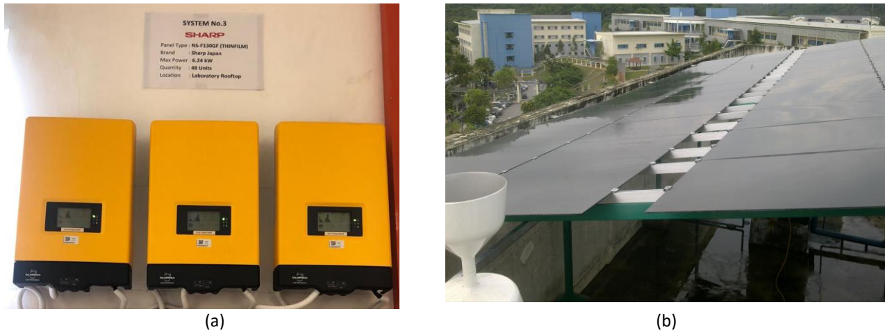
Fig. 2. (a) 6kW inverters system and (b) Thin-film module of PV system installed at FKE rooftop, UTeM
