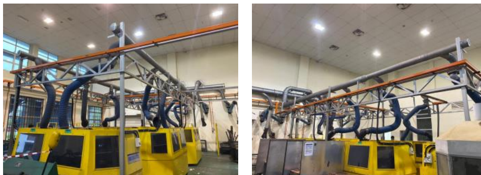
Fig. 1. Overview of LEV at Welding and Metal Fabrication Laboratory, FPTV
