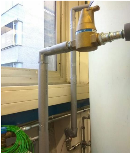
Fig. 4. Extension hydraulic setup area
