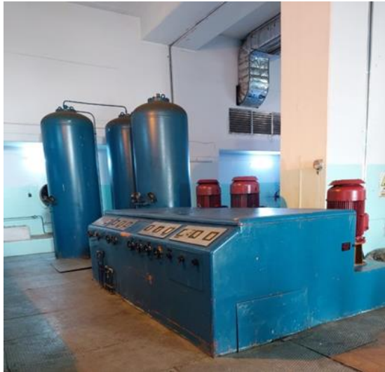
(c) The accumulators
