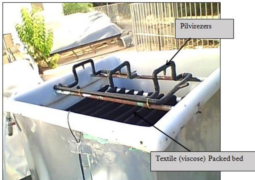
Fig. 4. Humidifier used in the solar desalination system
