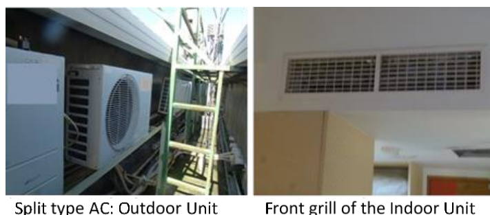
Fig. 2. Split AC system applied for Building-1
