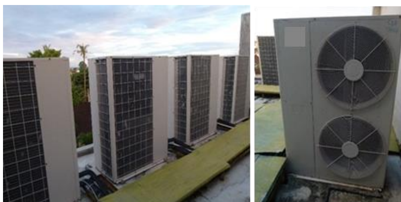
Fig. 4. The outdoor units of split AC systems for convention center
