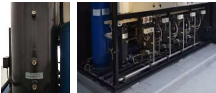
Fig. 4. The receiver tank sight glass at the compressor rack
