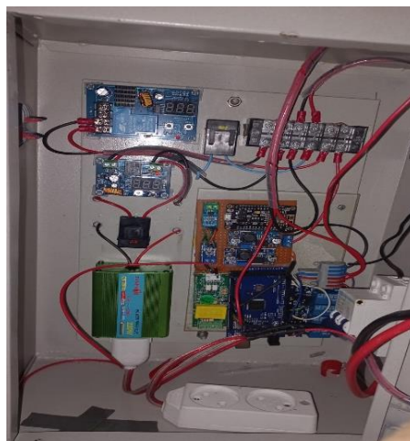
Fig. 5. Hardware control box of the microhydro power generator
