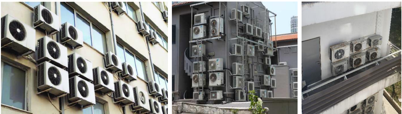
Fig. 9. Shows how HVAC systems were irregularly installed on the building facade spoiling its visual appeal
