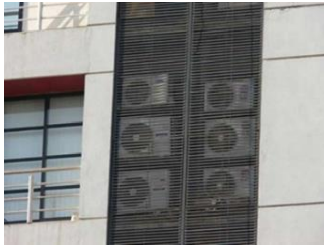
Fig. 17. Shows how the special space designed initially from the design phase enhances the overall building's aesthetics preventing AC chaotic façade
