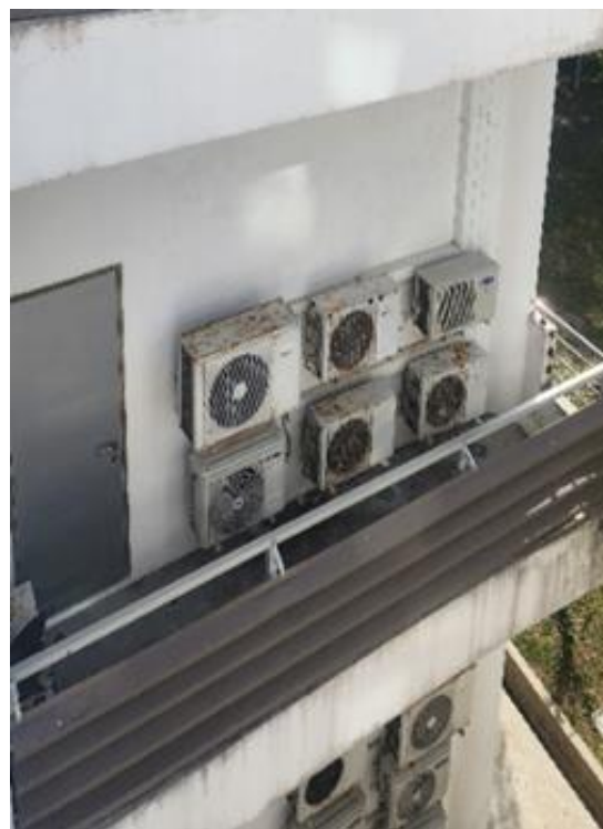
Fig. 18. Shows the example of HVAC systems installed on balconies that are subjected to solutions in Figure 22 and 23
